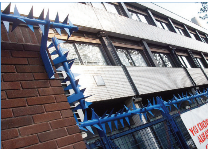
Security Rota Spike along building and fence run
