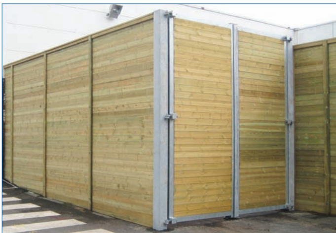
Small double leaf gate for access to waste compactor
