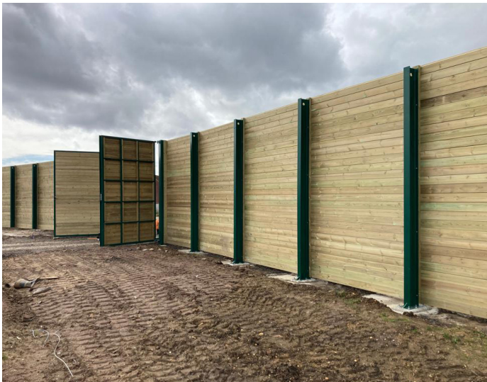
3.5m high acoustic barriers supported by steel I beams
