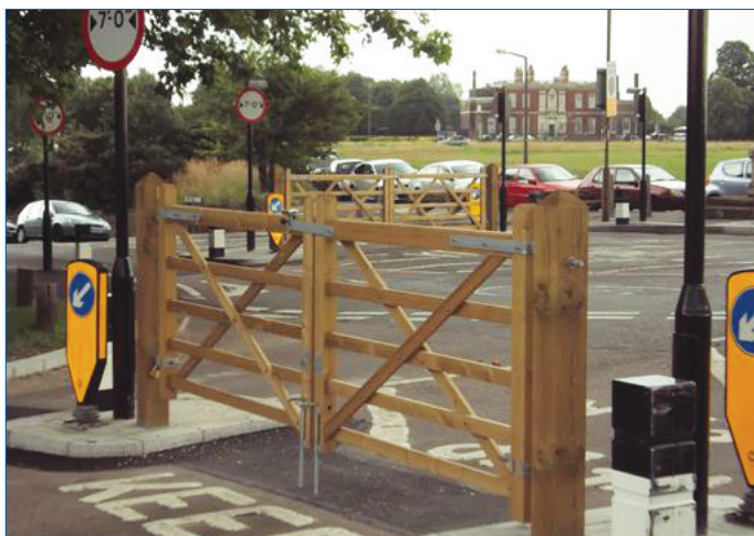
A double installation of new emergency gates in one location
