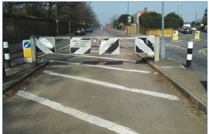
The old metal emergency gates were obviously in need of replacement
